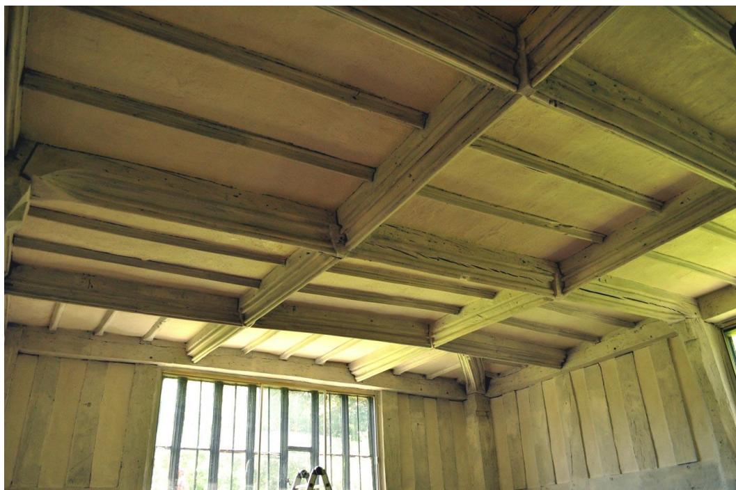
Figure 11. Eyton Court, Eyton, Herefordshire. The ground-floor ceiling beams, looking towards the diagonal dragon beam in the south-west corner.
