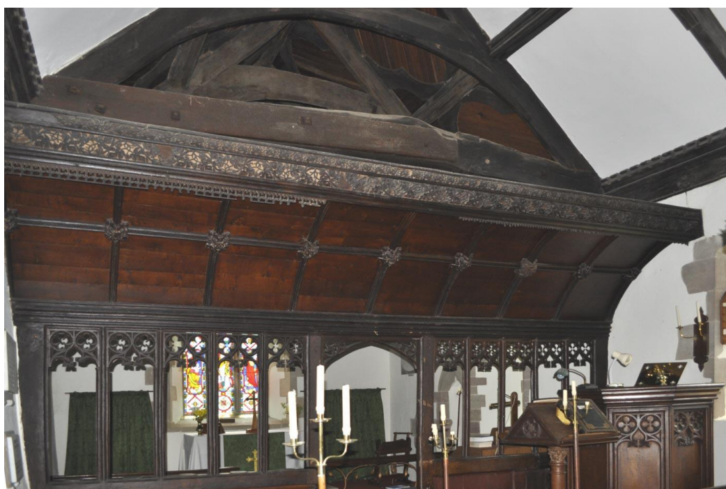
Figure 17. All Saints Church, Eyton, Herefordshire showing the early 16 th century screen with carved bosses and ribbing.
